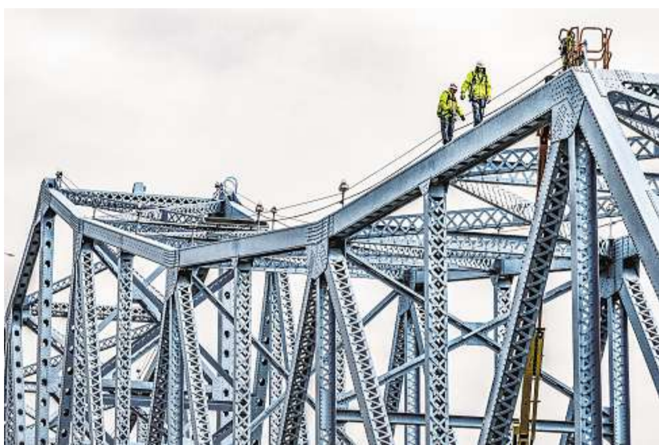
HIGH-WIRE ACT: Workers begin installing lights on the Owensboro Bridge, which spans the Ohio River between Indiana and Kentucky.
